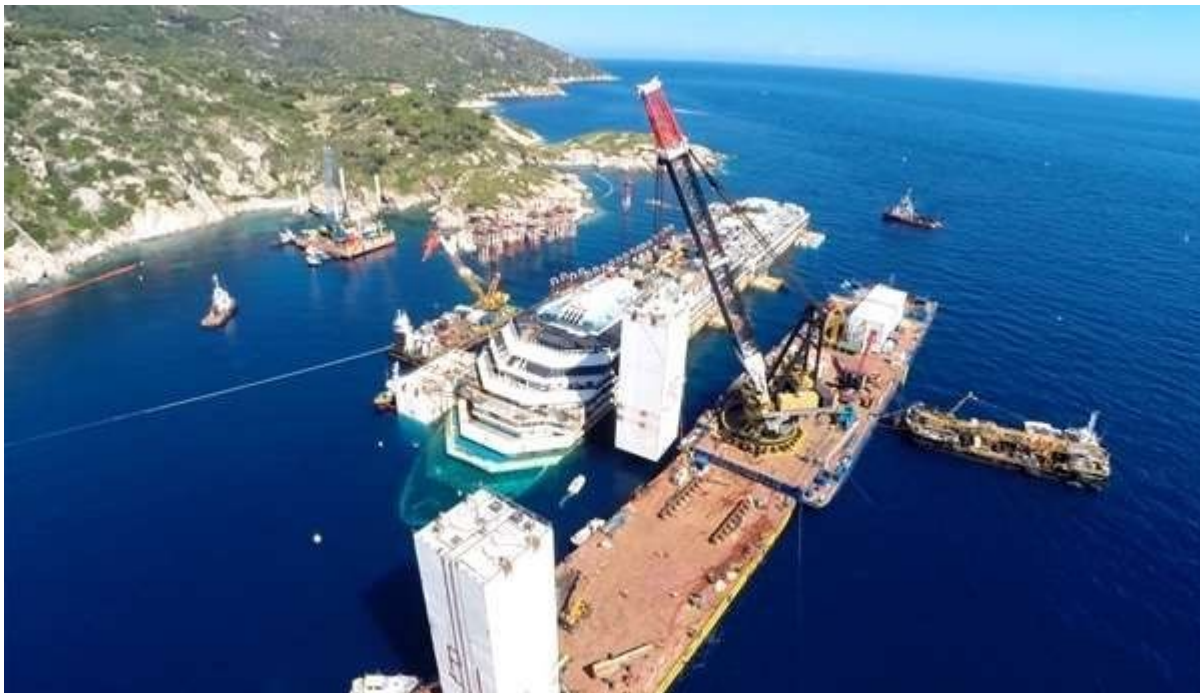
Installation of 850 ton buoyancy tanks on Costa Concordia, Italy 2014, using crane barge MB1.
